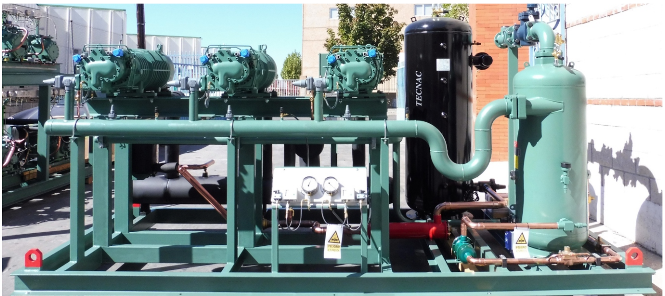
CENTRAL DE TORNILLO DE 3 COMPRESORES BITZER HSK: ACPT 3 X HSK7451-70 (-10/+45°C) R449A, Pot f= 309 kW
